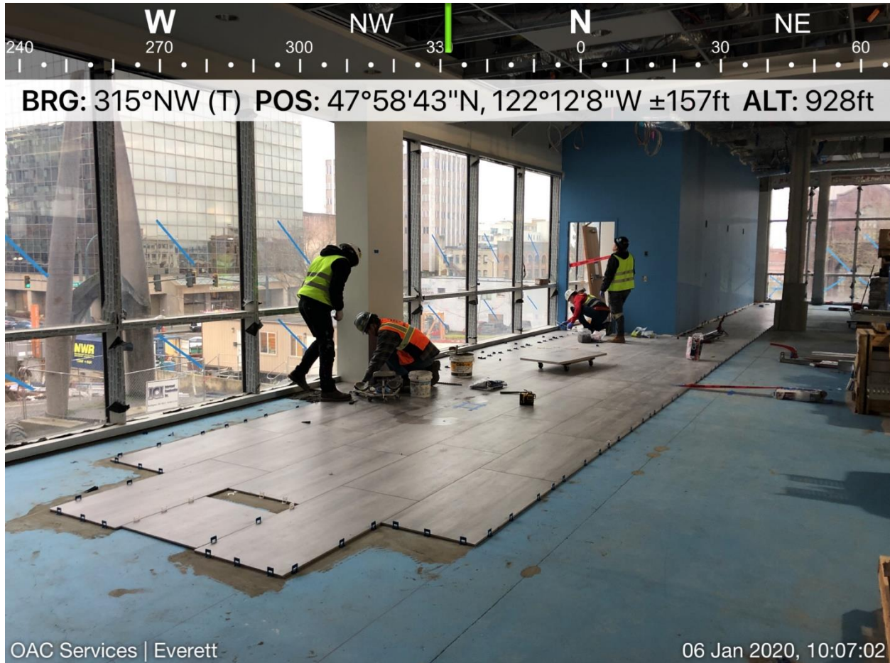
Flooring installation in the future Entry / Screening Area, Addition Level 1, viewed looking northwest from the vicinity of the Marshals' Station.
