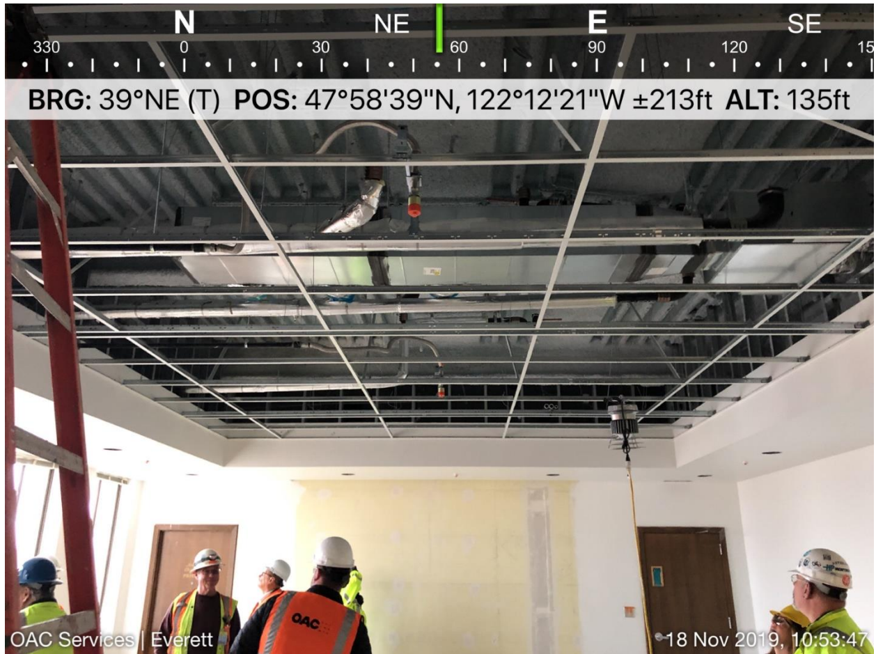
Soffits, ceiling grid, HVAC, and fire sprinklers in Courtroom 3A (District Court Dept. 2), looking straight east from the back of the gallery toward the bench area.
