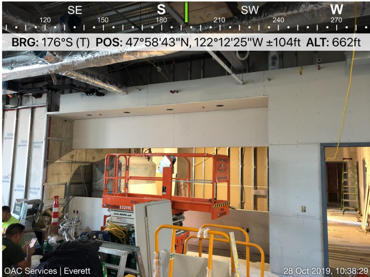
Future District Court Clerk Customer Service Center, as viewed looking southeast from the open office area to the north of the service counter.
