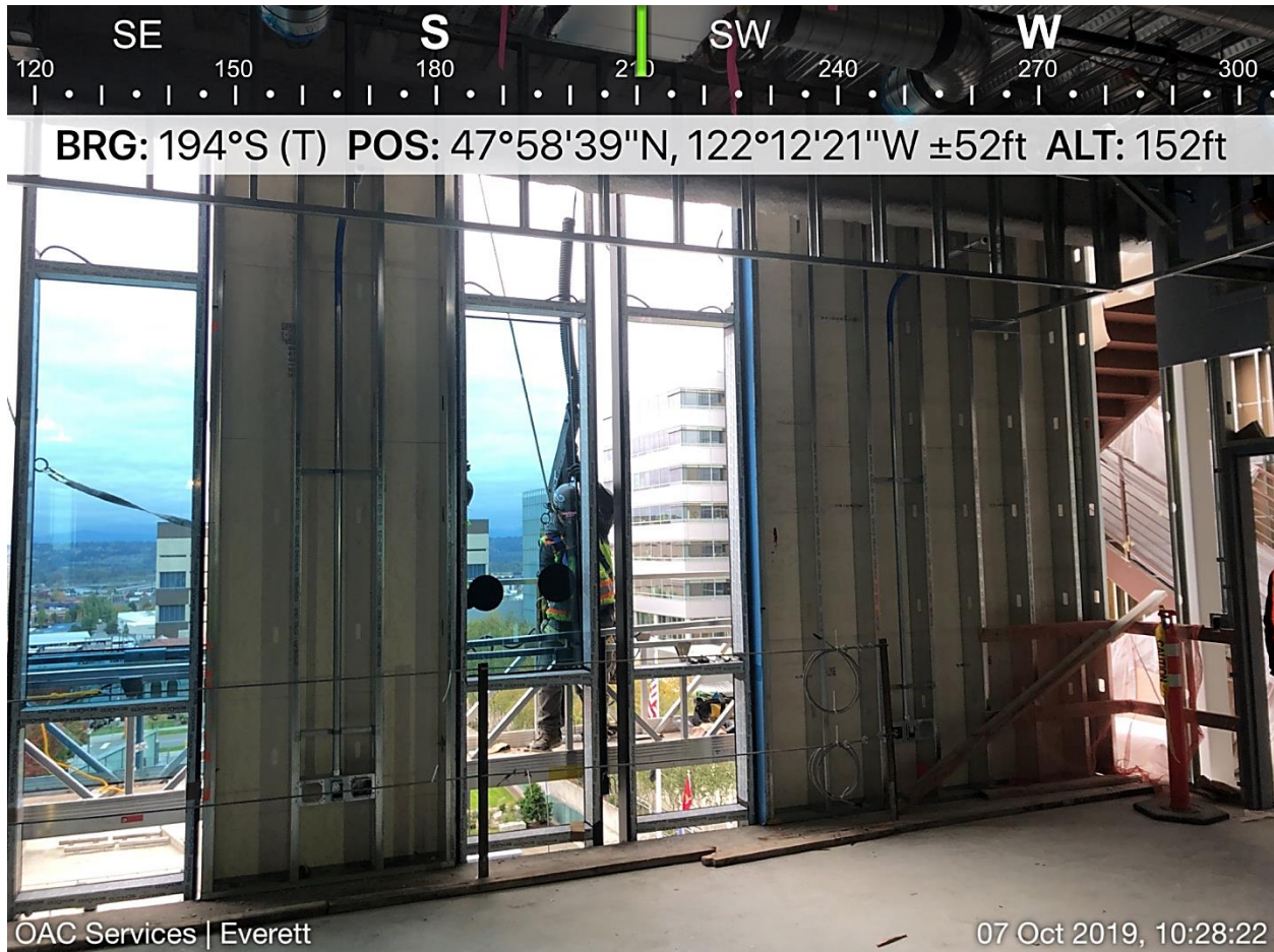
Installation of glass on the east face of the Addition at Level 3.
