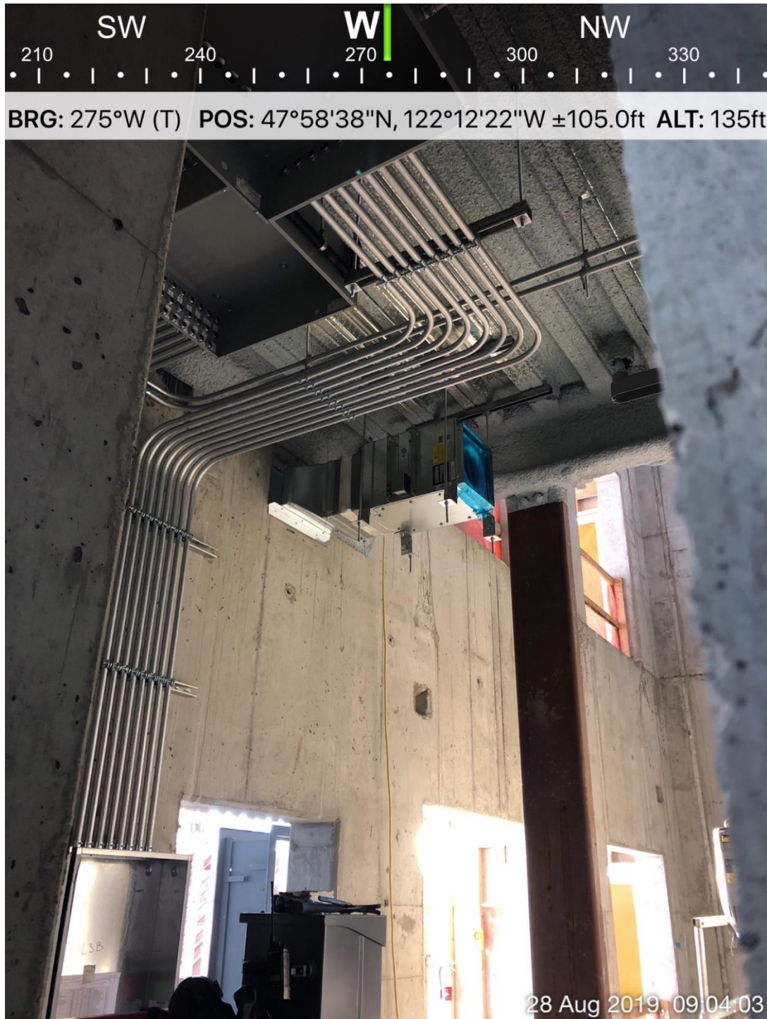
Electrical room on Addition Level 3, adjacent to the new elevator shaft.
