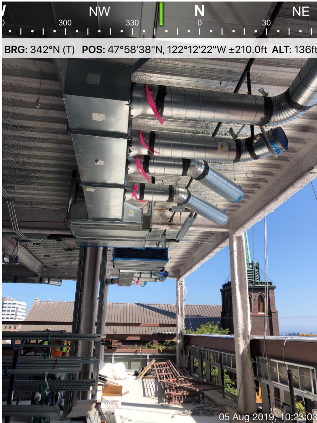
Overhead ductwork, with fireproofed structure and pan decking behind it, on Addition Level 2. The area shown will be the east end of the future Jury Assembly Room.
