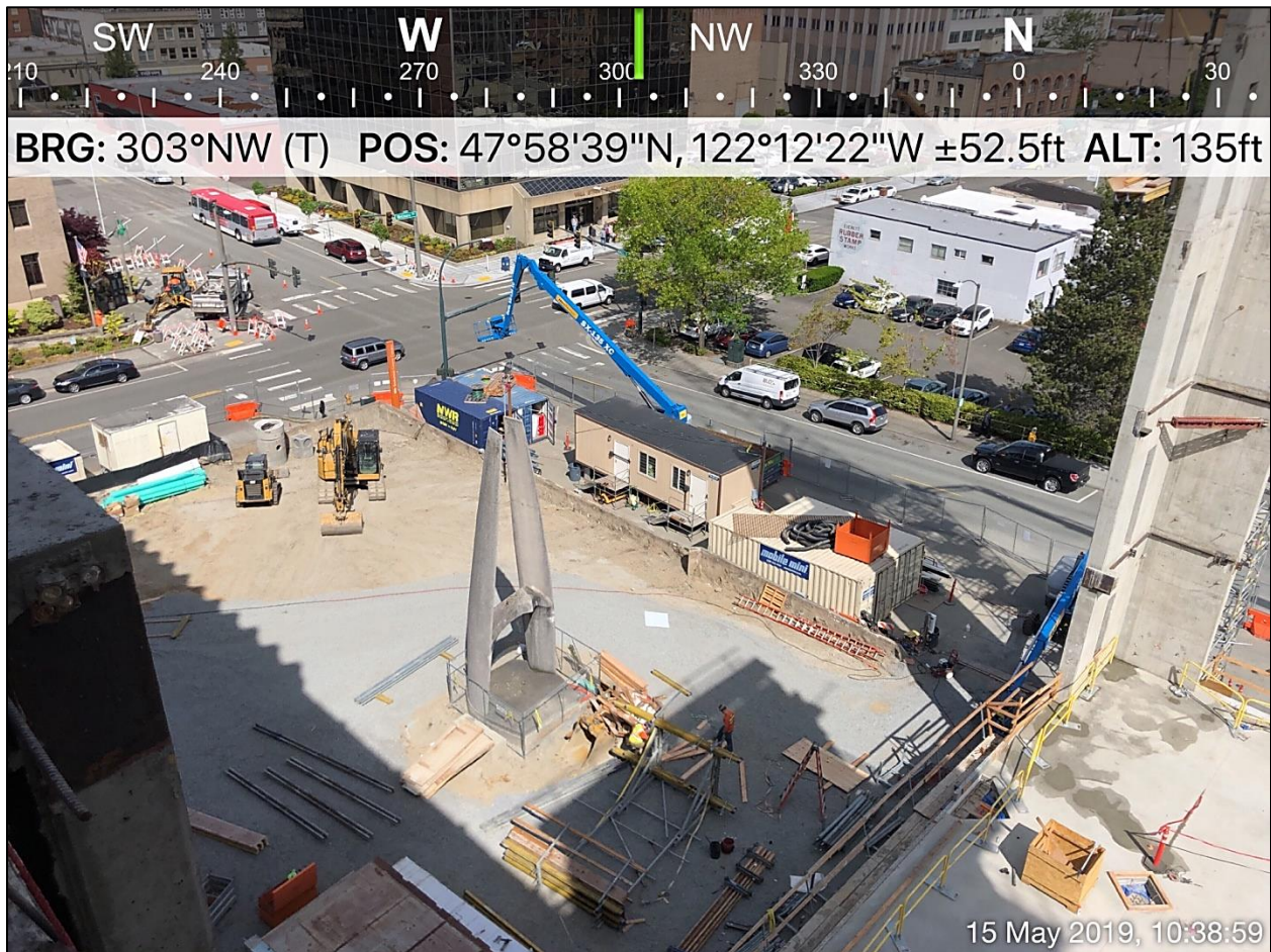
Site re-grading progress to date on the Northwest Plaza, as viewed from the north wall of the Courthouse. Addition slab-on-grade and northwest shear wall are at the far right of the photo.
